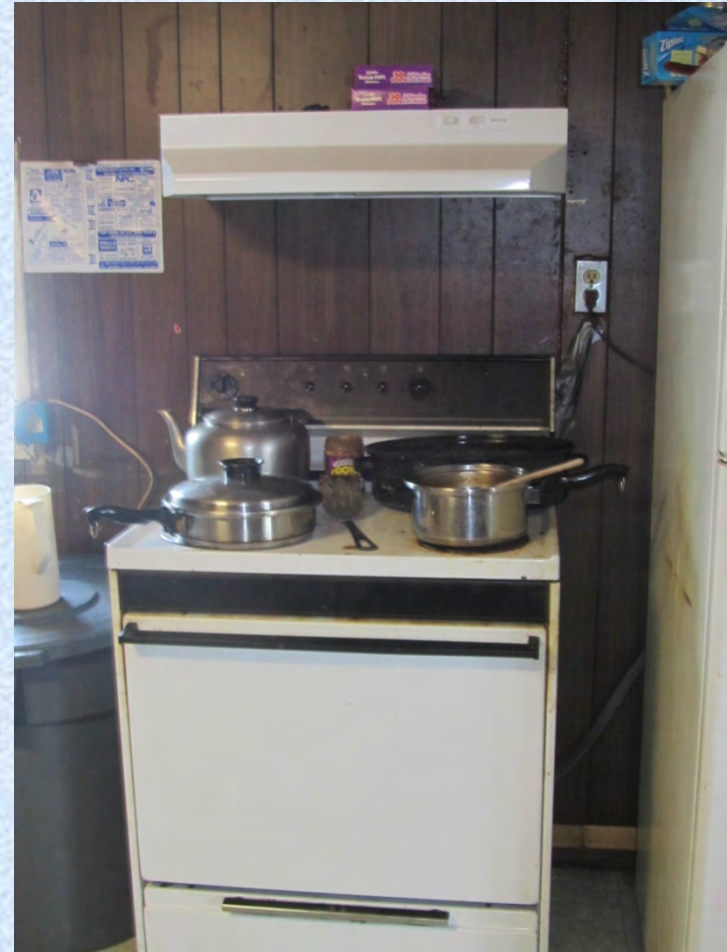
Cooking stove with a new range exhaust
