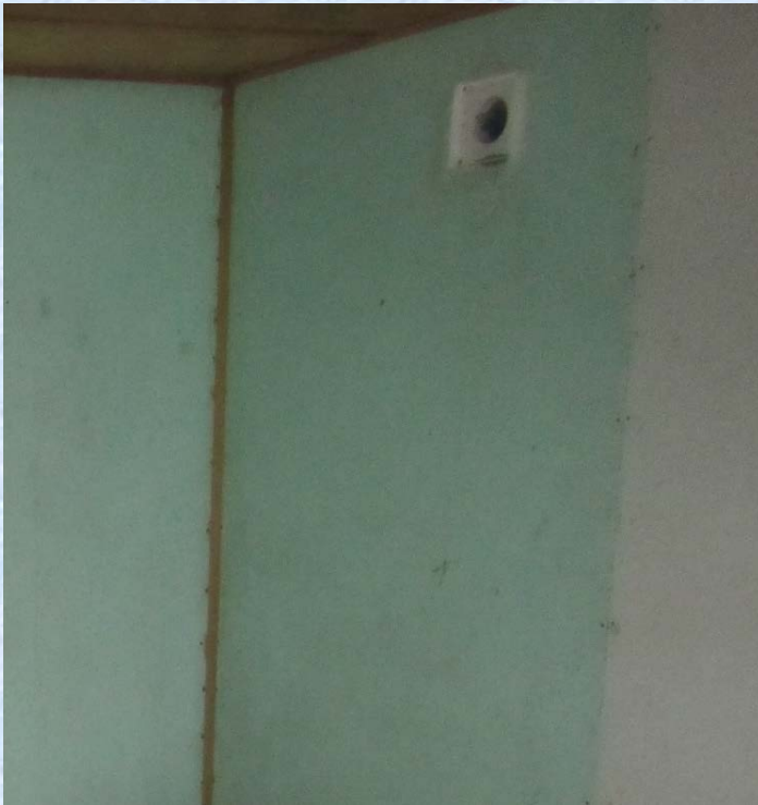
Ventilation intake plugged with a rag
